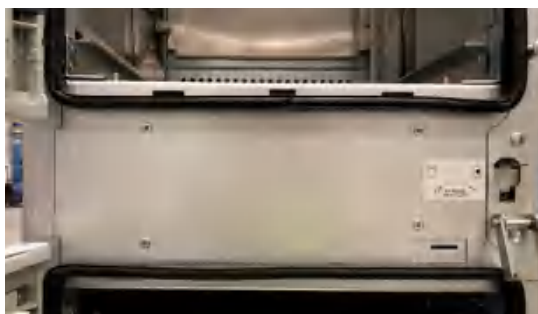
Figure 47 Front view on window among cable and circuit - breaker compartment
