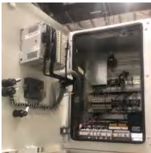
Figure 7 Low-voltage compartment, internal view
