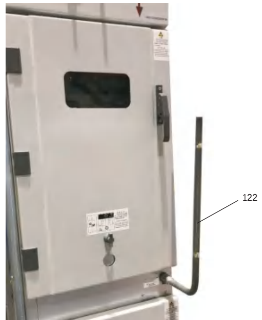
Figure 70 Preparing to operate the earthing switch - operating lever in upright position ready to switch to on/off position
