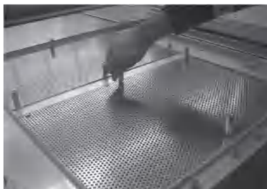
Figure 57 Net and spacers of top chimneys
