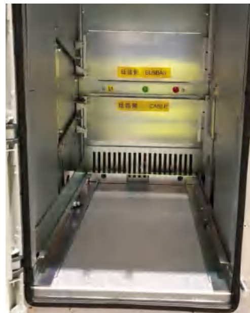
Figure 48 Circuit- breaker compartment
