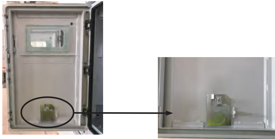
Figure 8 Circuit- breaker compartment door enabling device
