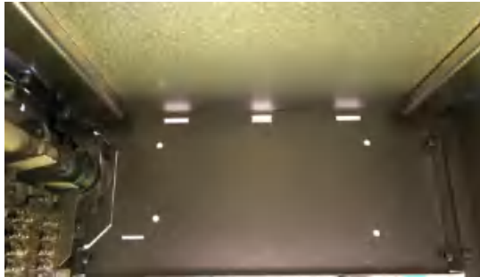
Figure 45 View from cable compartment
