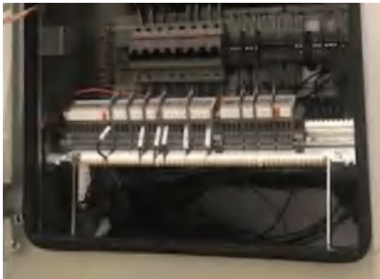
Figure 60 An open terminal frame
