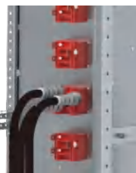
Form4b cable connection with separation
