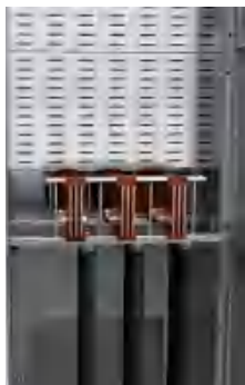
ACB Cable connection
